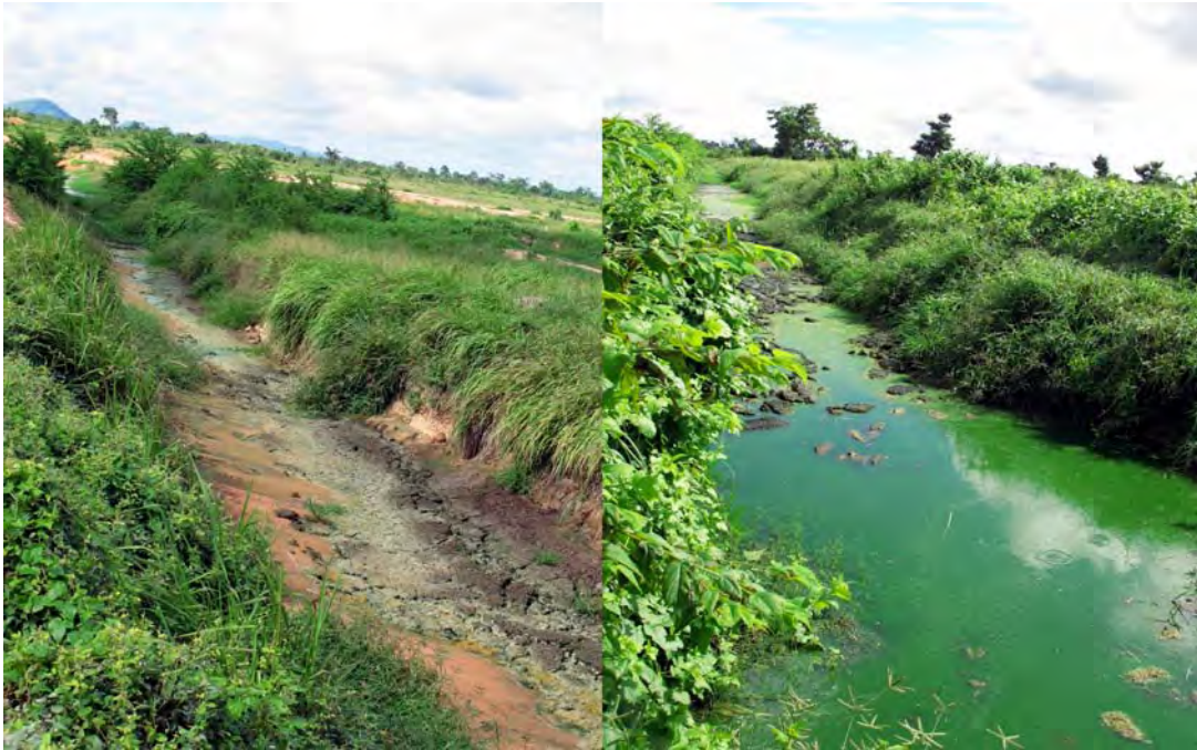
Traces of waste water in emptied canal (left) and canal still filled with waste water mixed with rain (right) on company land, June 2010.
